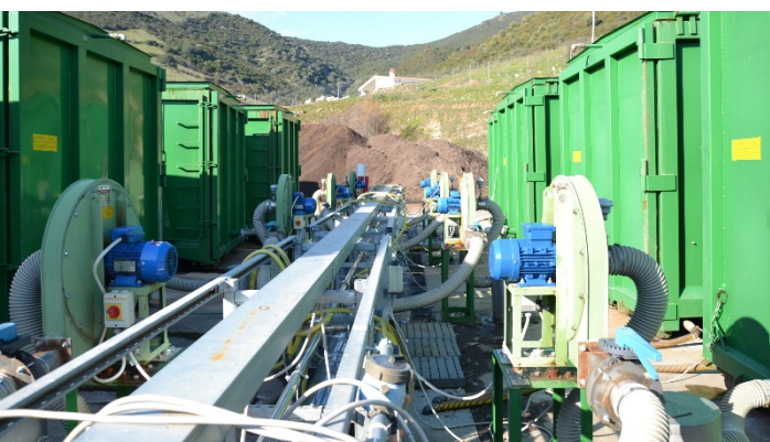
1. AUTOMATIC FORCED VENTILATION SYSTEM
